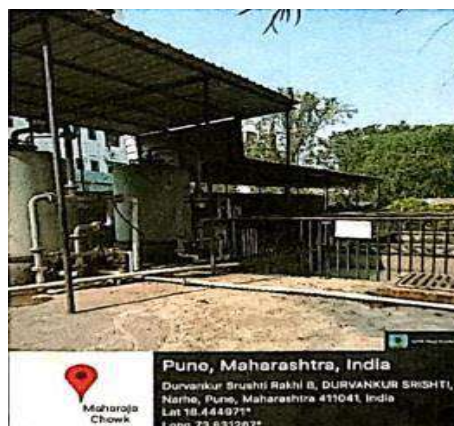
Photographs of sewage treatment plant
