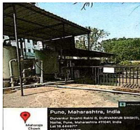
Photographs of sewage treatment plant
