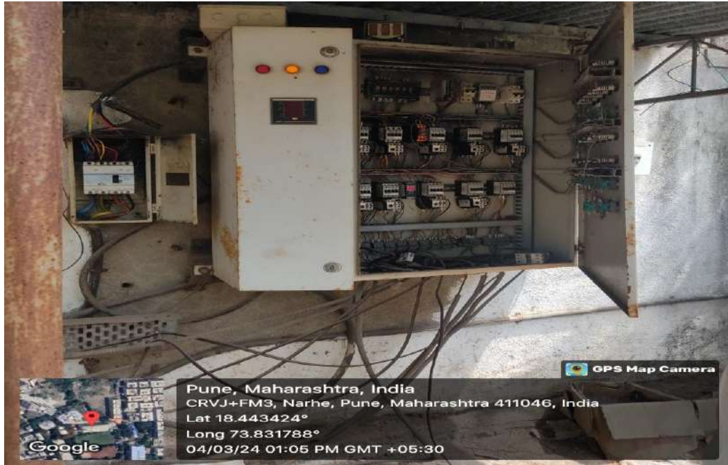
Automation panel for water recycling
