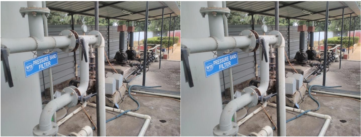
Fig. 1 Sewage Treatment Plant
